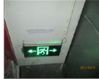
Photo of fire safety equipment Evacuation indicating sign.JPG
