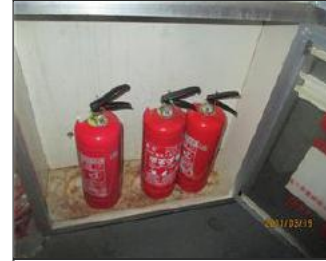
Photo of fire safety equipment Fire extinguishers.JPG
