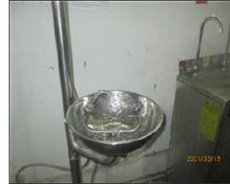
Photo first aid facilities Eye washing station.JPG
