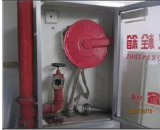
Photo of fire safety equipment Fire hydrant.JPG
