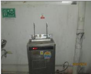
Photo of the sanitary facilities Drinking water area.JPG
